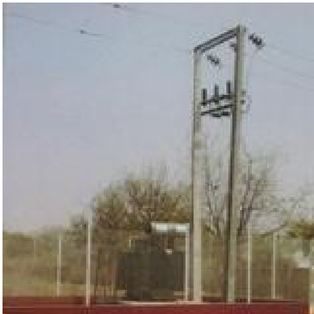
Extension of 33KVA to Federal Polytechnic, Damaturu, Yobe State
